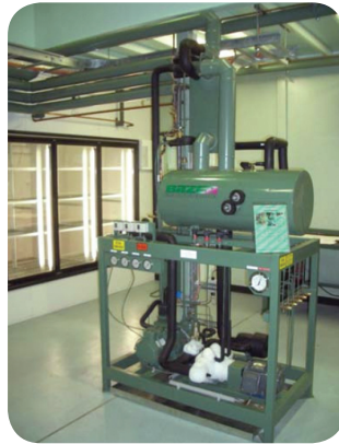
Picture 6 – Rack for sub-critic operation with CO 2 using recirculation pump for evaporators of medium evaporation temperature
