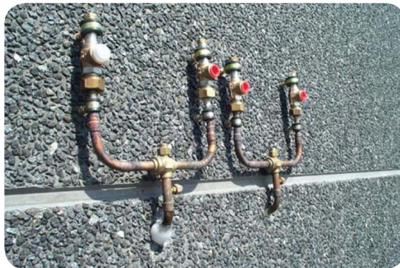
Picture 2 – Security valves installed in outside of machine room, “without tubing ending to avoid blockade for ice”
