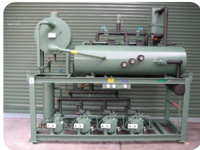
Picture 13 – Detail of tank of liquid mounted in a rack thermally isolated
