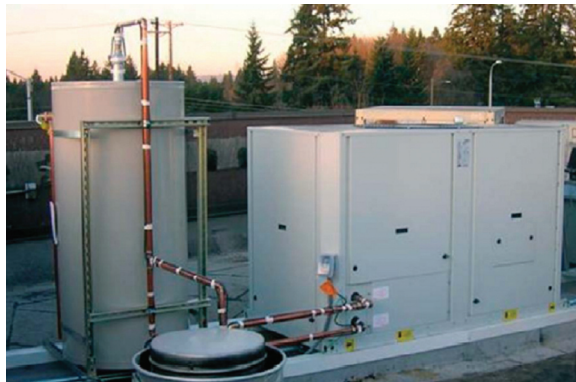
Figure 3 – Industrial 60kW CO 2 heat pump water heater (T. Seinel, IEA v.24.3.2006)
