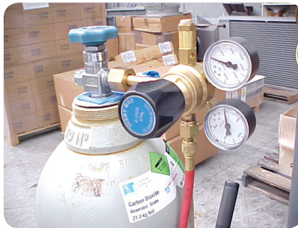
Picture 7 – Detail of regulator pressure valve installed in CO 2 cylinder
