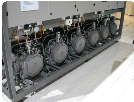
Picture 3 – Rack with transcritical application of CO 2
